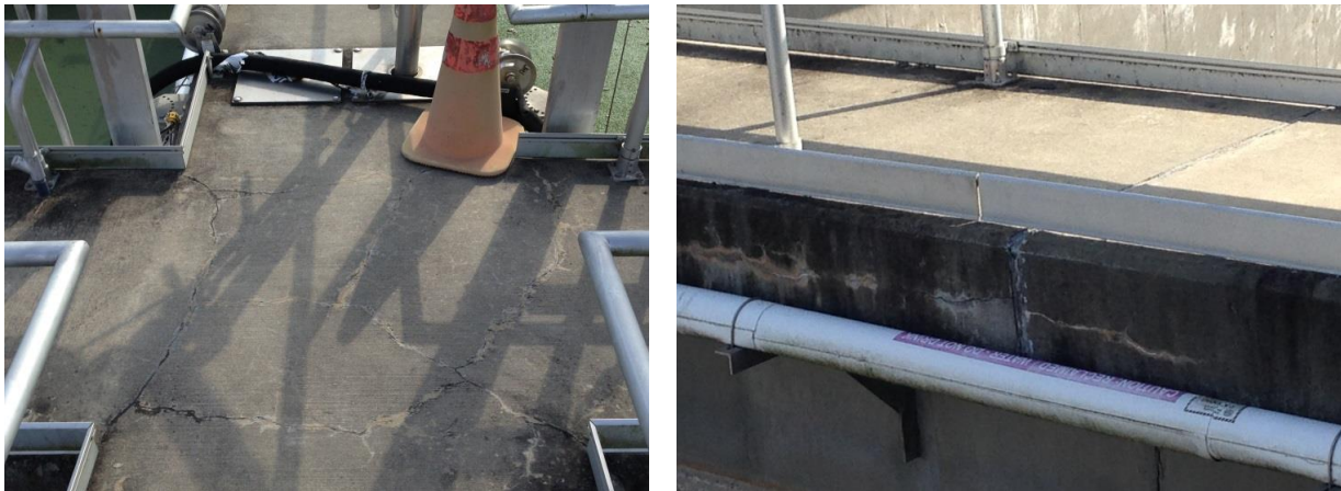
Figure 5-1: Existing Cracking in Walkway
