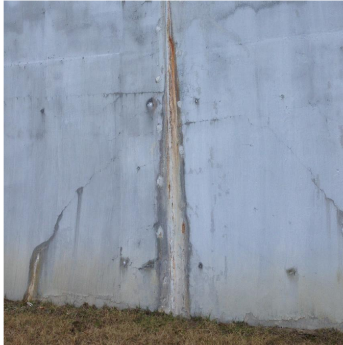
Figure 5-2: Efflorescence at Expansion Joint.
