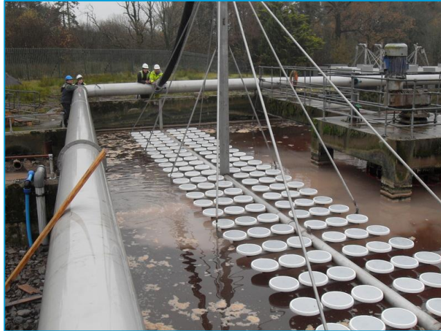
Figure 3-4: Example Installation of a Retrievable Diffuser System
